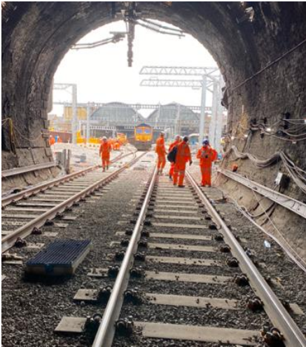
Sicut Plastic Composite Sleepers installed in the London Kings Cross Gasworks Tunnel
